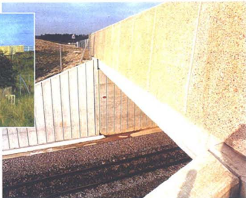
Precast concrete parapets with exposed aggregate finish shown over the London-Pentance railway.
