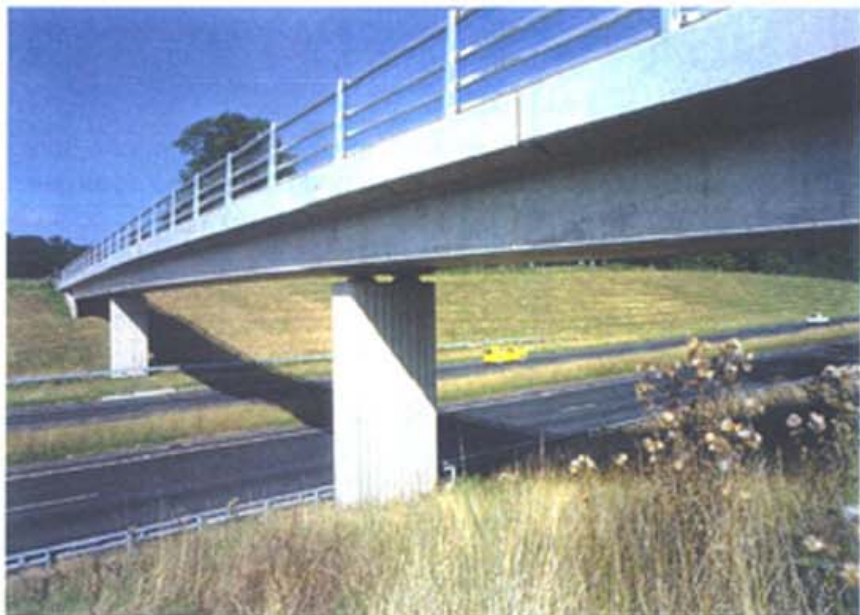
High slag content concrete enhanced the finish and gave a uniform colour.
